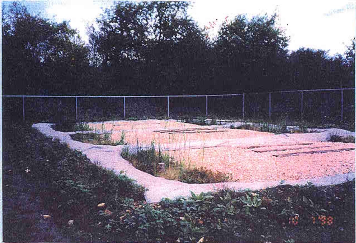
Figure 7. Commonwealth Edison railway tie mesocosm study site in the Fall of 1998, approximately six months following construction.
